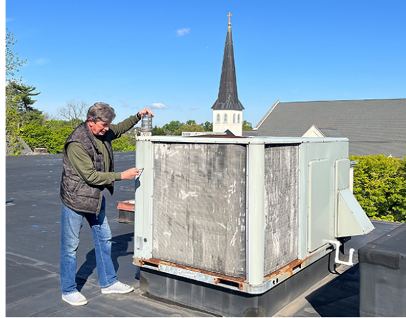
HVAC units will be repaired or replaced.
